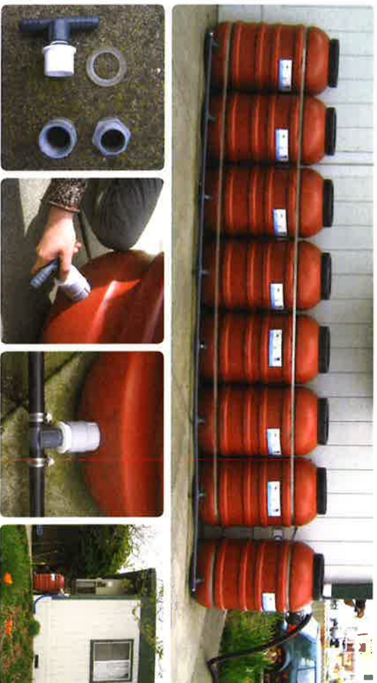
A daisy-chained system of the SFPUC's Southeast Wastewater Treatment Plant.
