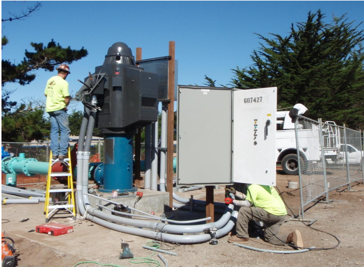
Final electrical connections to new well
