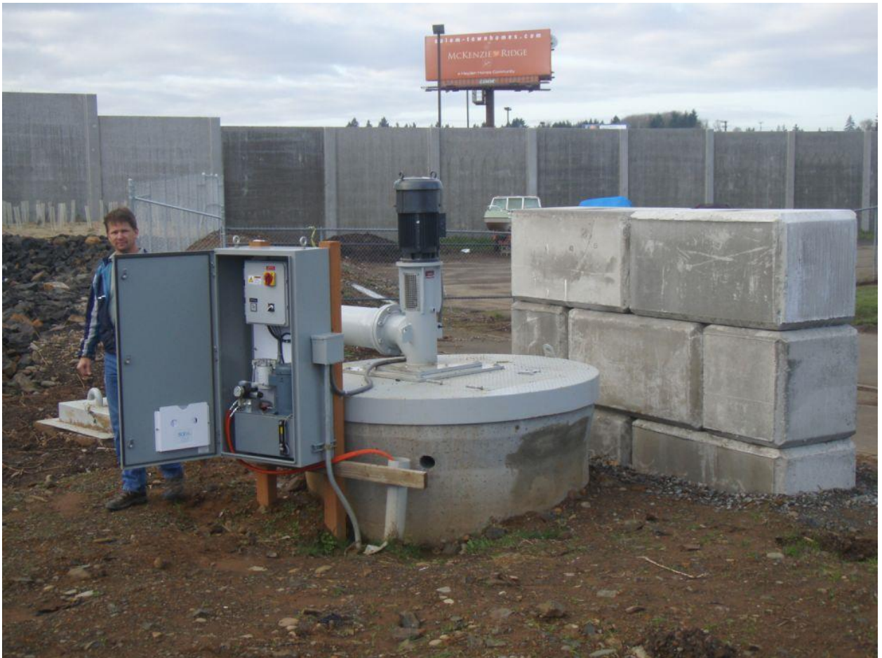
Image 3- Example of pump motor and electrical supply raised out of wet well to improve access.
