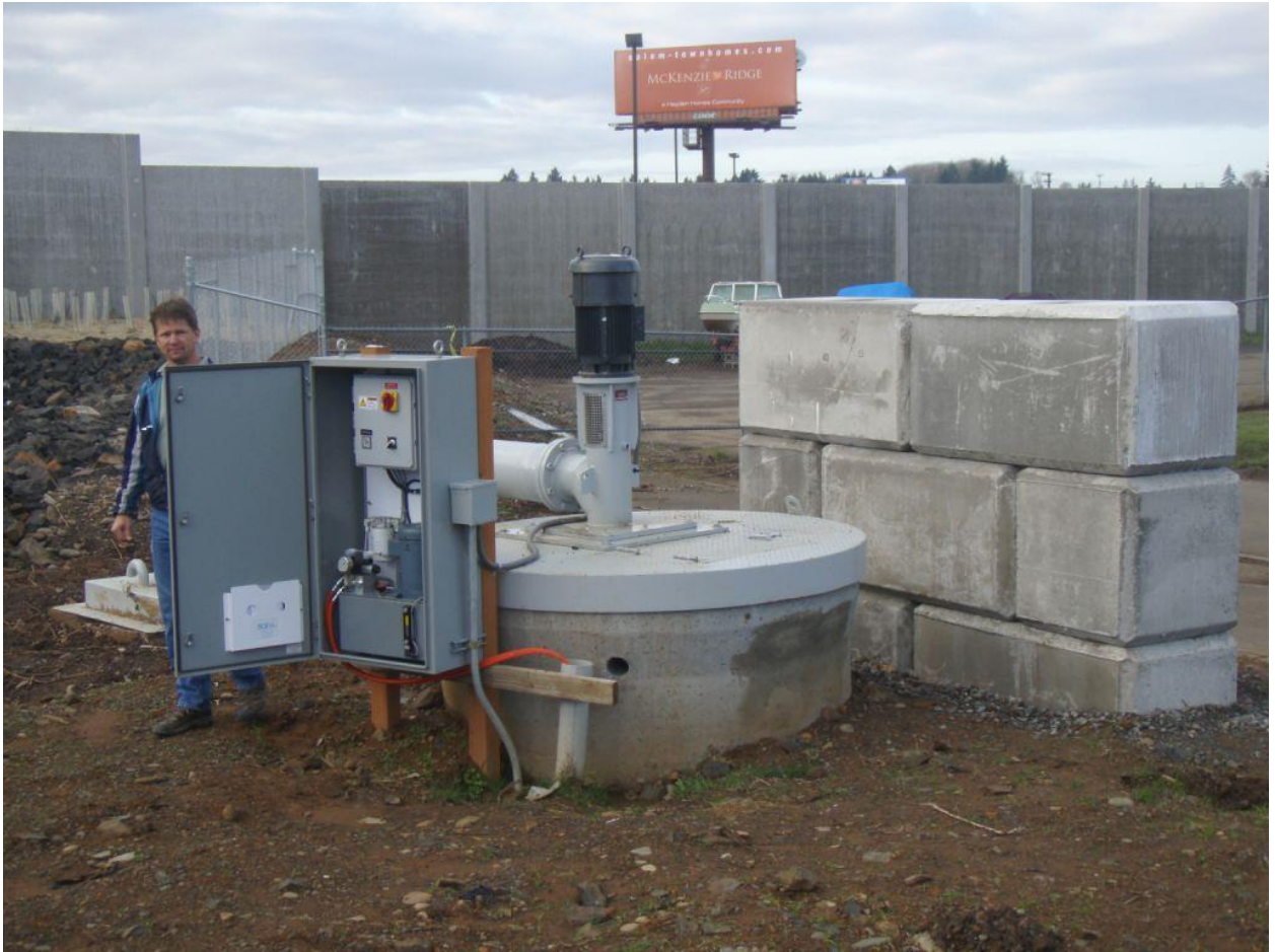
Image 3- Example of pump motor and electrical supply raised out of wet well to improve access.
