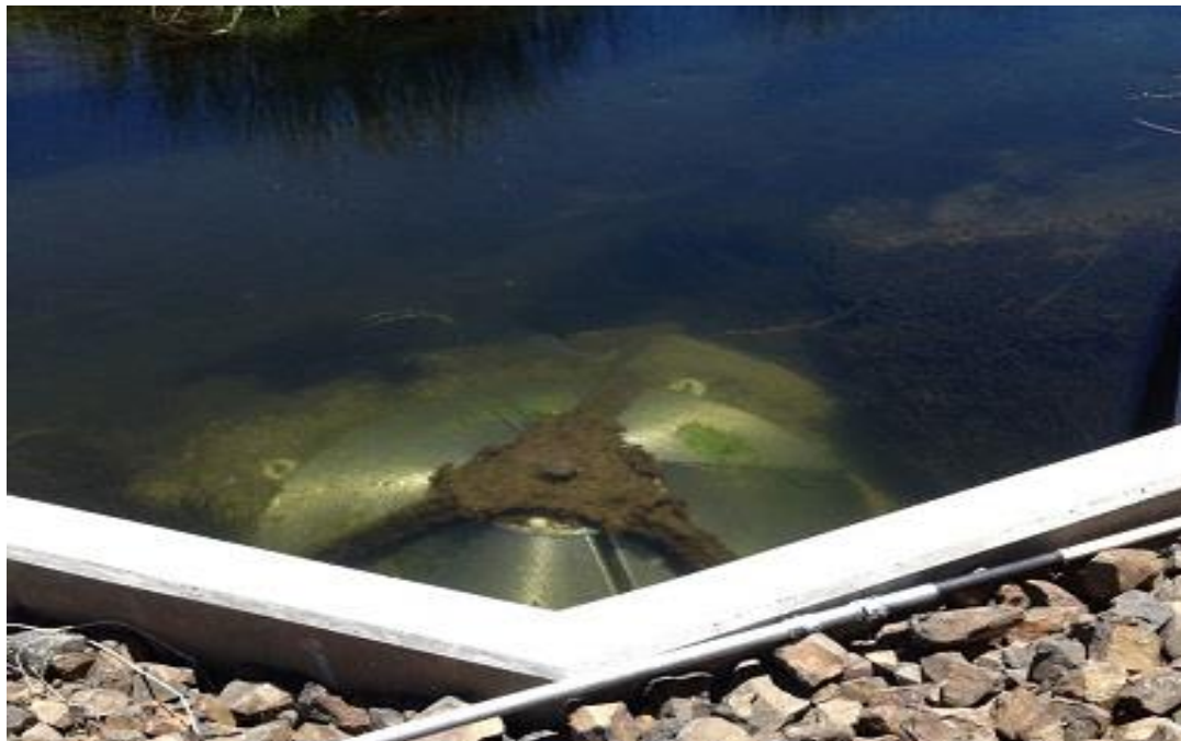
Image 2- Example of cone screen underwater in an alcove with external cleaning brushes in operation.
