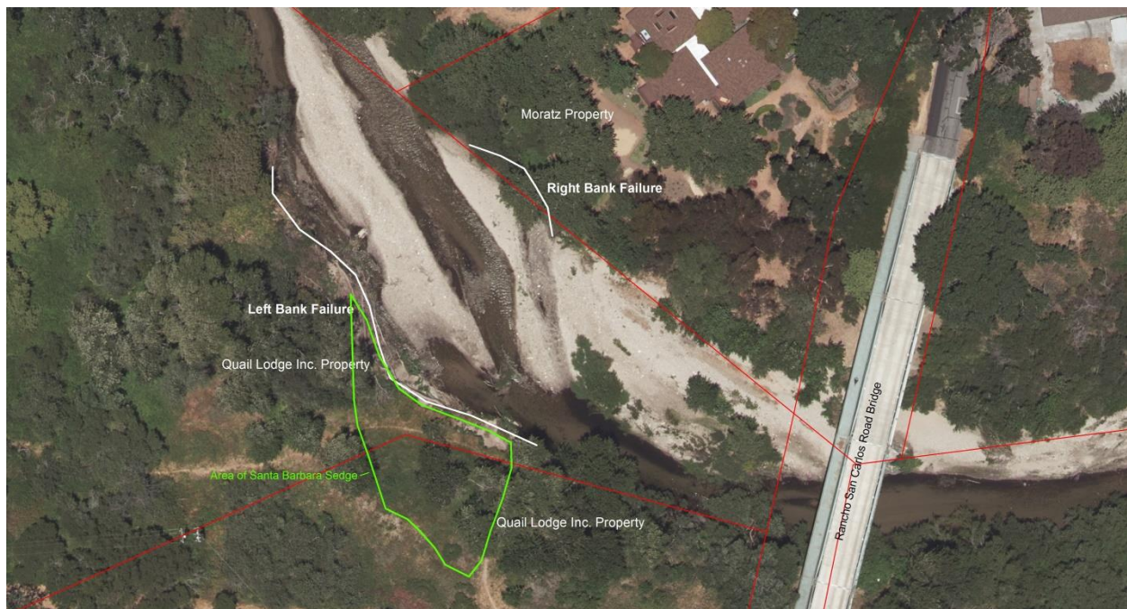
Figure 3. Aerial image showing locations of erosion just downstream of Rancho San Carlos Road Bridge
