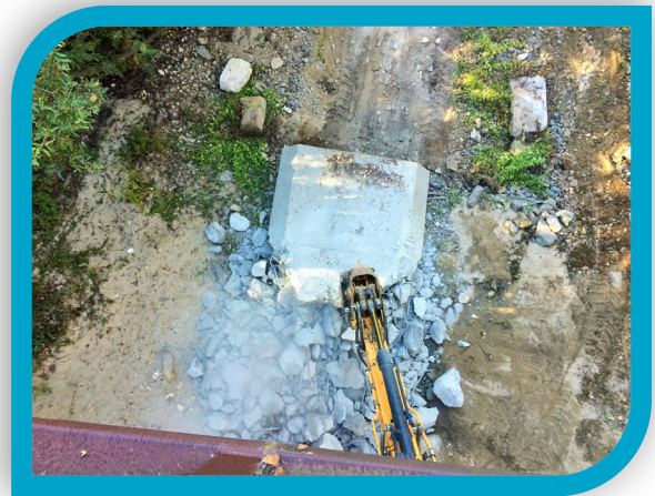
View from above, as District staff use a hoe ram to remove a concrete bridge pier lying in the Carmel River.
