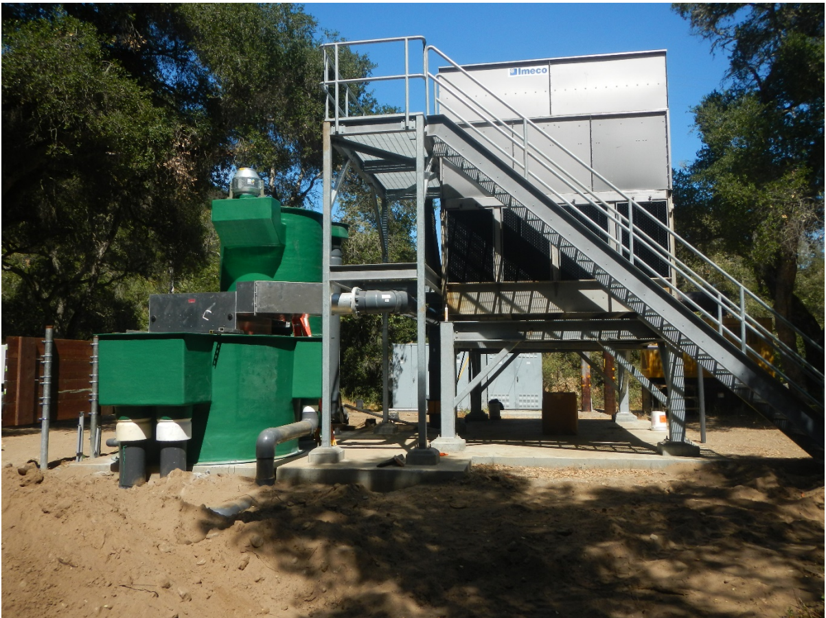
(Photo: Sleepy Hollow Colling Tower & Tank)
