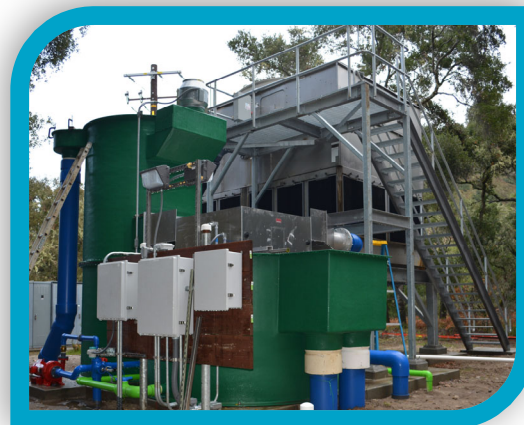
New construction at Sleepy Hollow Steelhead Rearing Facility. When the upgrade is completed the facility will operate during periods of extreme drought or high flows and should be operational for the 2020 fish rescue and rearing season.
