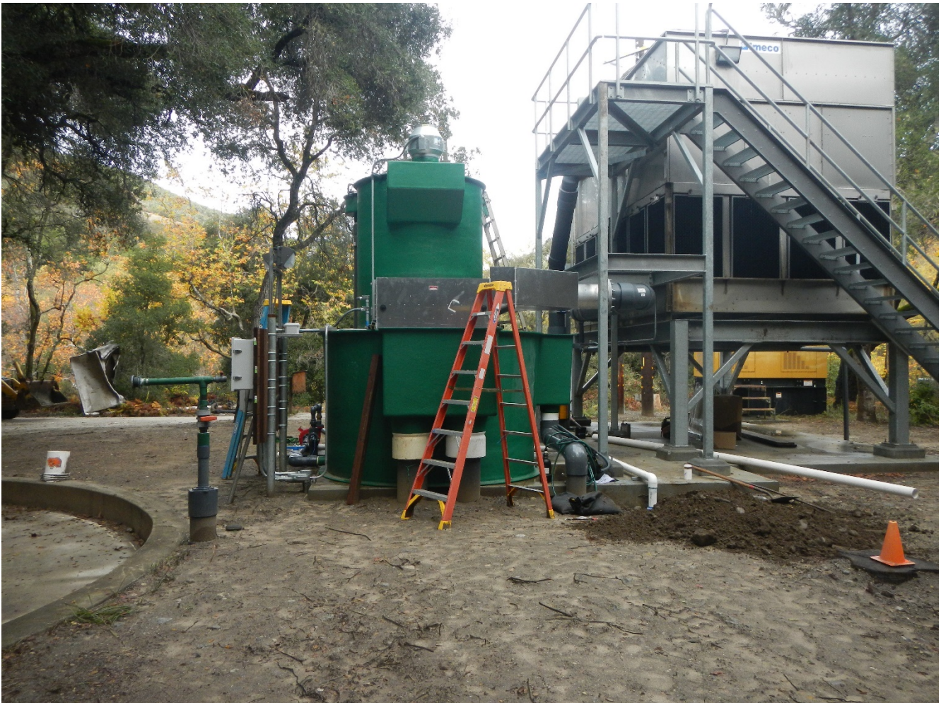
(Photo: Sleepy Hollow Cooling Tower)
