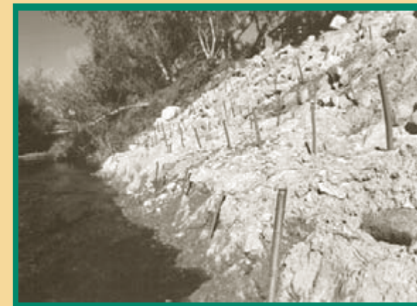
Neighbors must cooperate to create a continuum of bank protection. This bank restoration project shows newly planted willow cuttings taking root. With irrigation during dry periods, these fast-growing native trees will provide a high level of bank protection in just a few years, while at the same time increasing aesthetics, wildlife habitat, water quality and property value.
