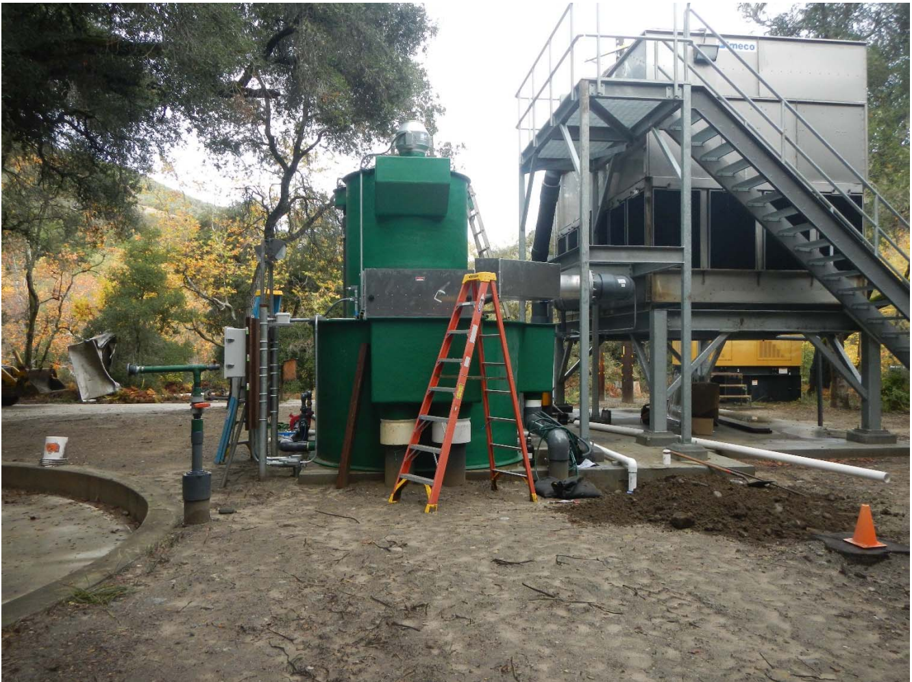
(Photo: Sleepy Hollow Cooling Tower)
